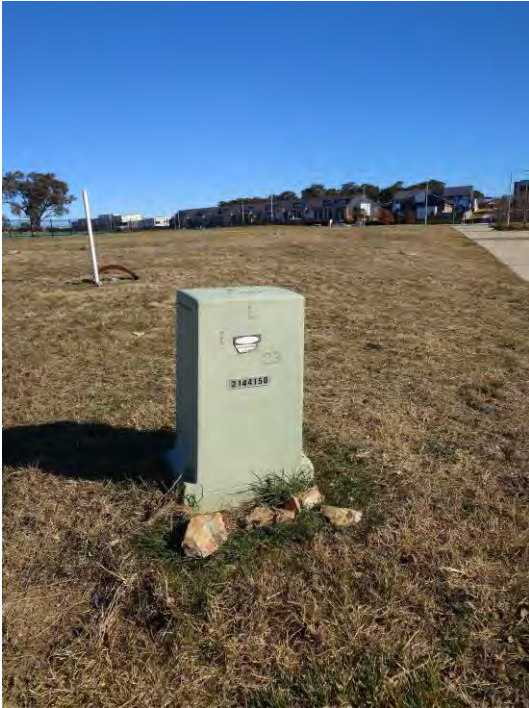
Figure 50 – Electrical Mini Pillar Near North East Corner of the Site
