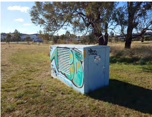
Figure 51 – Electrical Substation (S 11057) North East of the Site
