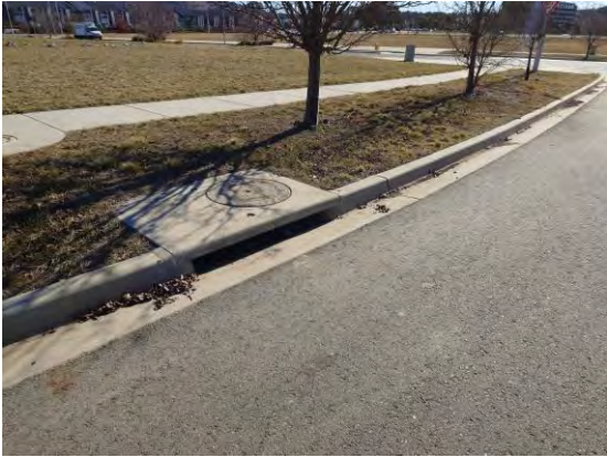
Figure 29 – Stormwater Sump in West Verge of Hoffmann Street East of Site
