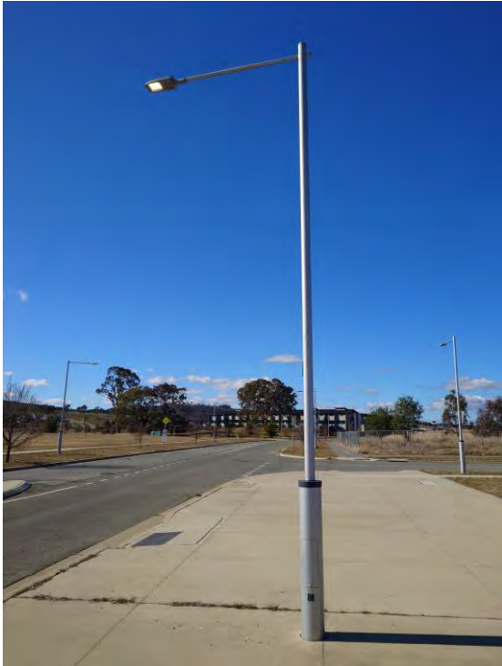
Figure 47 – TCCS Streetlights in O'Keefe Avenue
