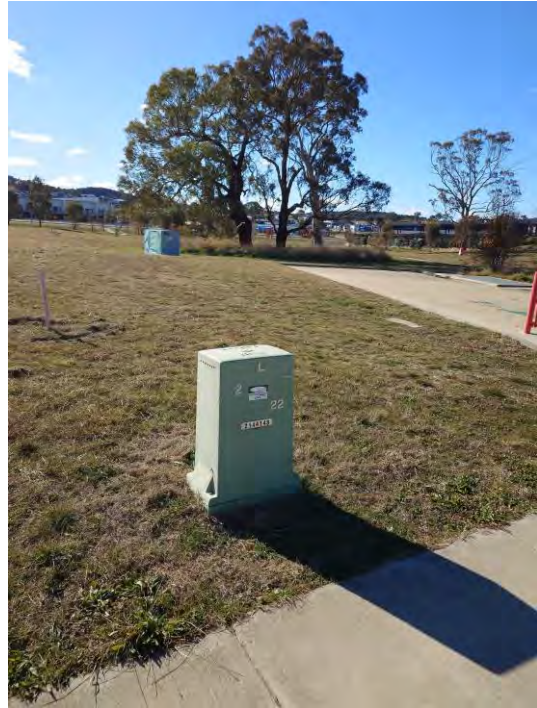
Figure 52 – Electrical Mini Pillar and Substation in Distance North East of Site
