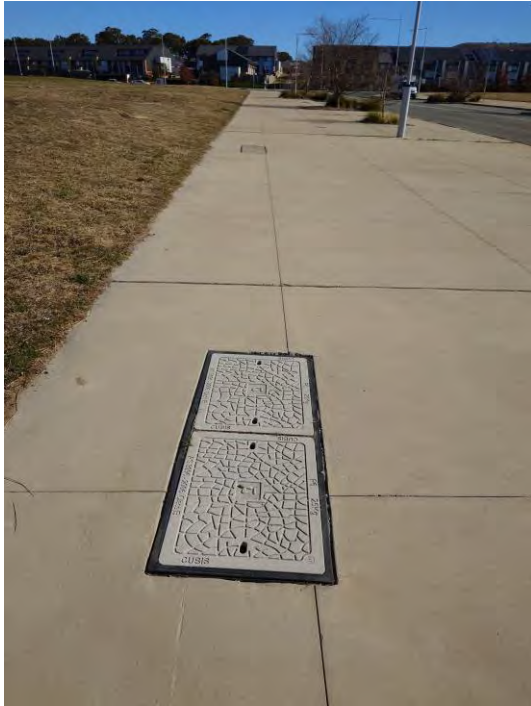
Figure 37 – Telstra Pit in Southern Verge of O'Keefe Avenue North East of Site
