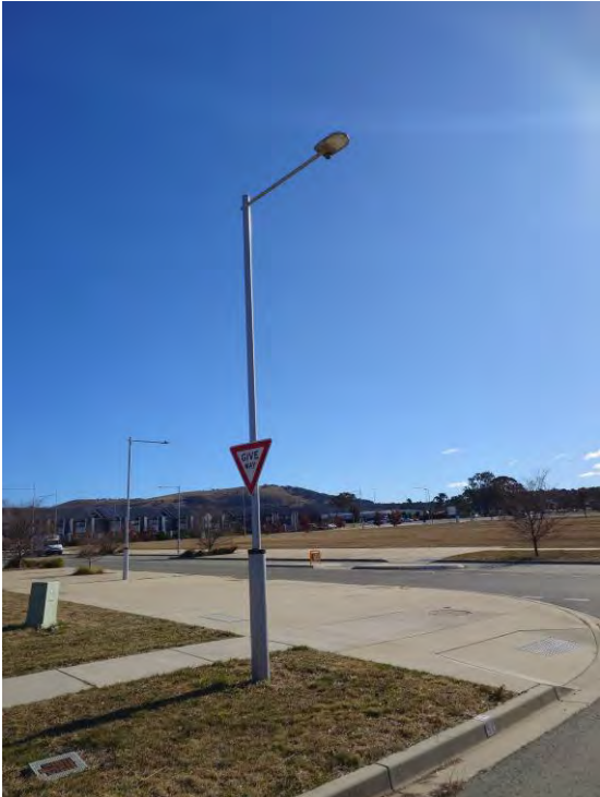
Figure 45 – TCCS Streetlight at Intersection of Hoffmann Street and O'Keefe Avenue
