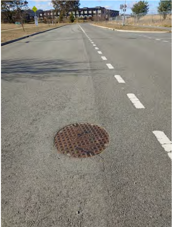
Figure 32 – Stormwater Manholes in O'Keefe Avenue North East of the Site
