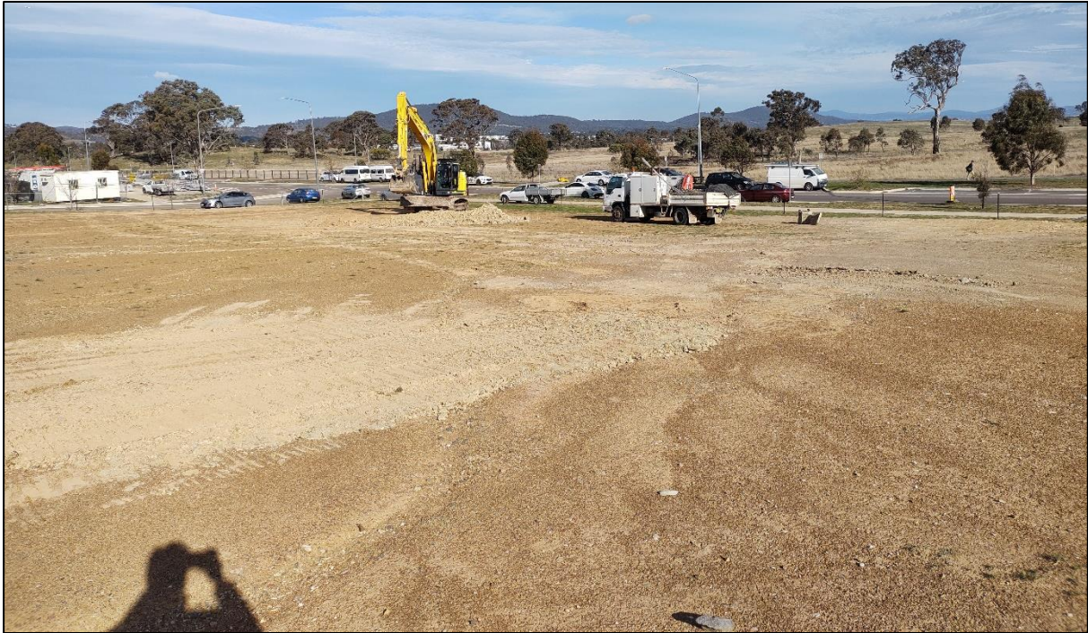
Figure 1: View looking south-east across the block, with the excavator located at Pit 3.
