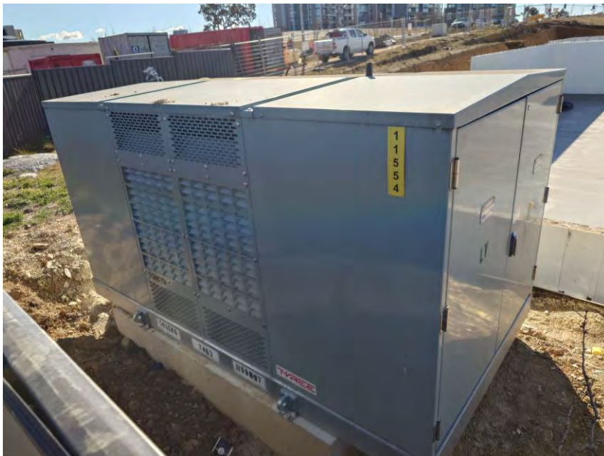
Figure 48 – Electrical Substation (S 11554) in South East Corner of Block 7 Section 249
