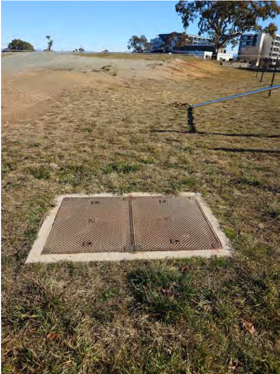
Figure 37 – Telstra Access Chamber North East of Site
