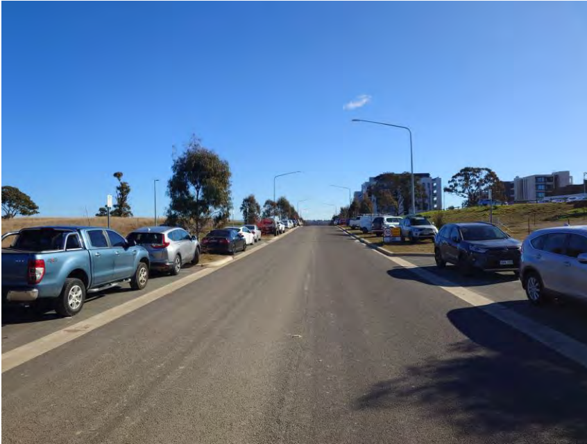
Figure 46 – Streetlights on Camilleri Way
