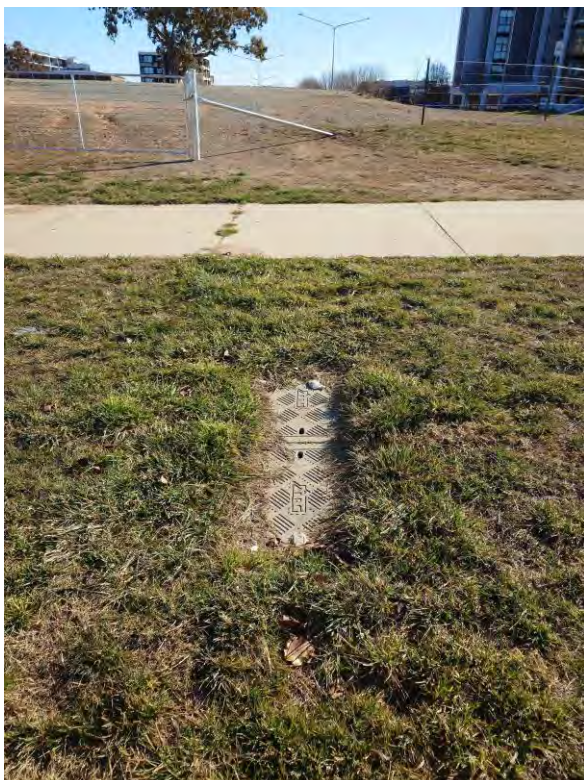
Figure 40 – TPG Pit in West Verge of Kate Grace Street North East of the Site
