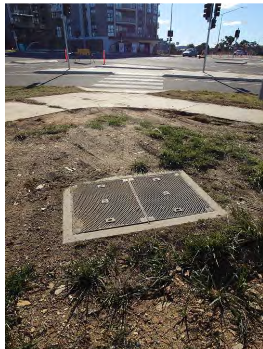
Figure 36 – Telstra Access Chamber North East of Site
